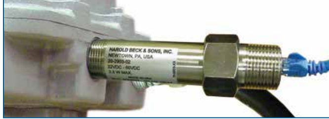
INSTALLED BECK MODBUS TCP ADAPTER
