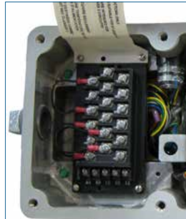
Field Wiring Terminals
